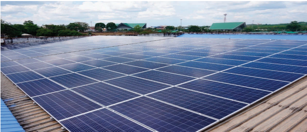
Solar Panel at Bukit Kayu Hitam Outlet
